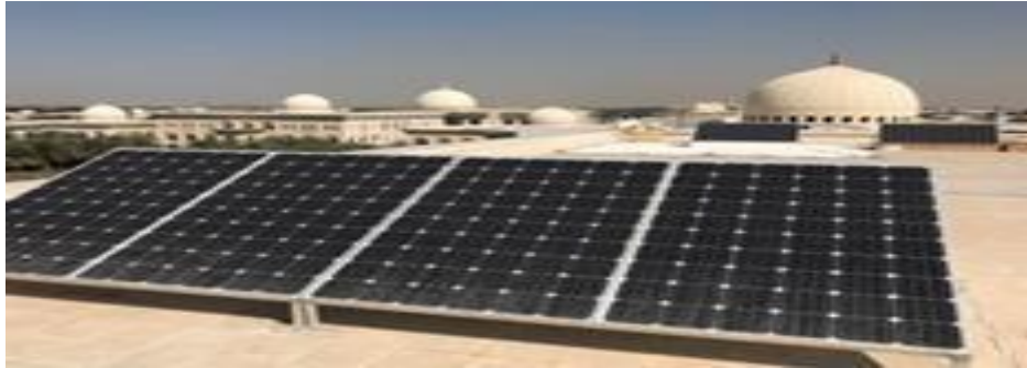
Figure 49: Solar system to power the greenhouse.
