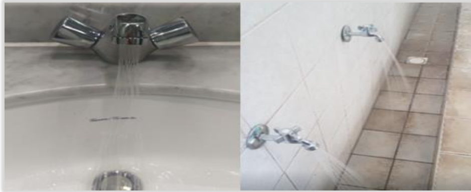
Figure 25: Water nozzles at washrooms.
